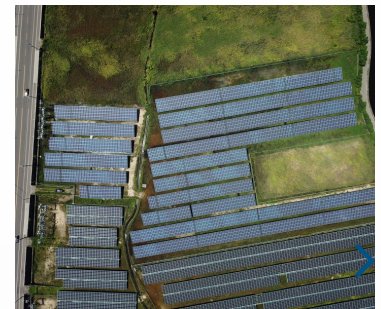
5MW Brubeck | Chiayi Budai Dongshi Power Plant
